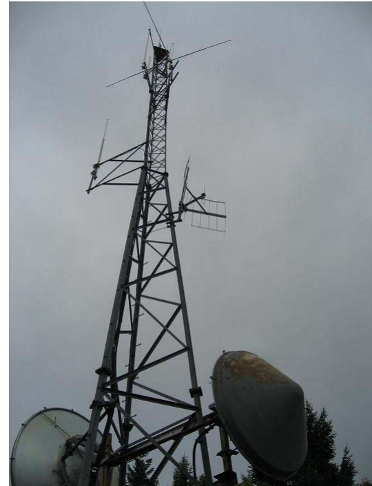
The radio tower at Hoadley Peak supports antennas as well as microwave dishes.
